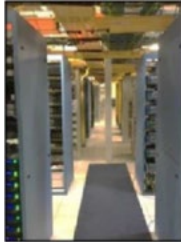
Interior Rack Spaces
