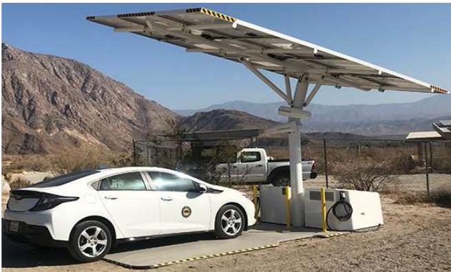
Off-Grid Solar + Storage
